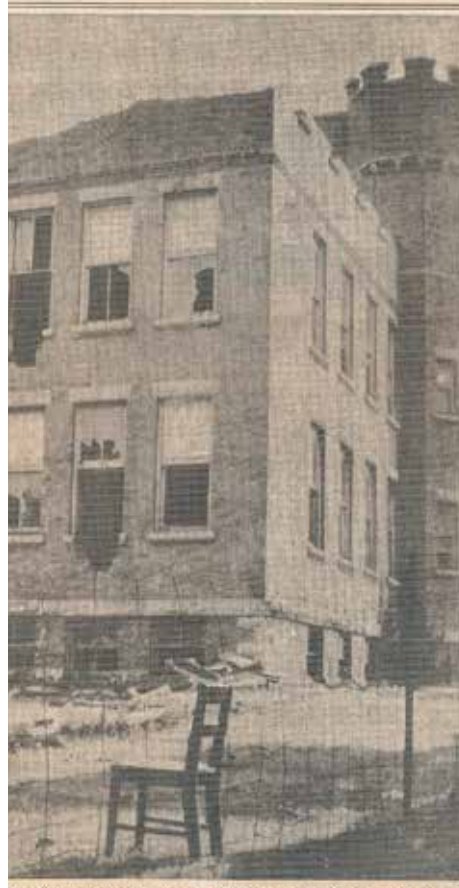
BUT NOT FORGOTTEN — The old Bellefontaine high school is taking on a dilapidated architecture as it crumbles under the stroke of a demolition crew, and it has been punched in its sides. Tuesday workers plan to move in a crane, fixed with a bucket, which will then pick the older section of the modernized building full of rubble. Trucks will haul it to its final resting place at a site along north Troy. The demolished will be the old auditorium, according to C. F. Williams, contractor. (Examiner Staff)
