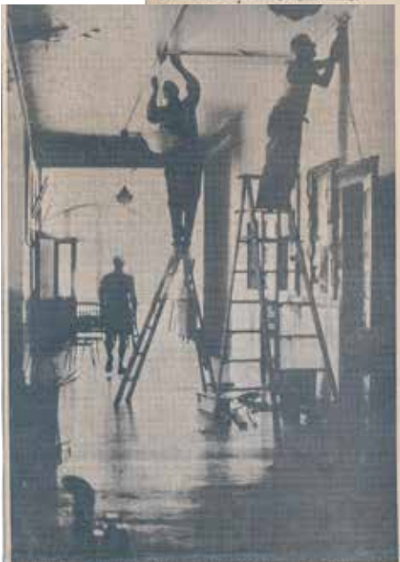
Electrician Homer Dugan, shown at the bottom of the ladder on the right, and some of his employees are shown as they strip wiring and light fixtures from the old middle school here Monday. The equipment will be moved for possible use in other buildings, he said. (Examiner Photo by Brown Scott)
